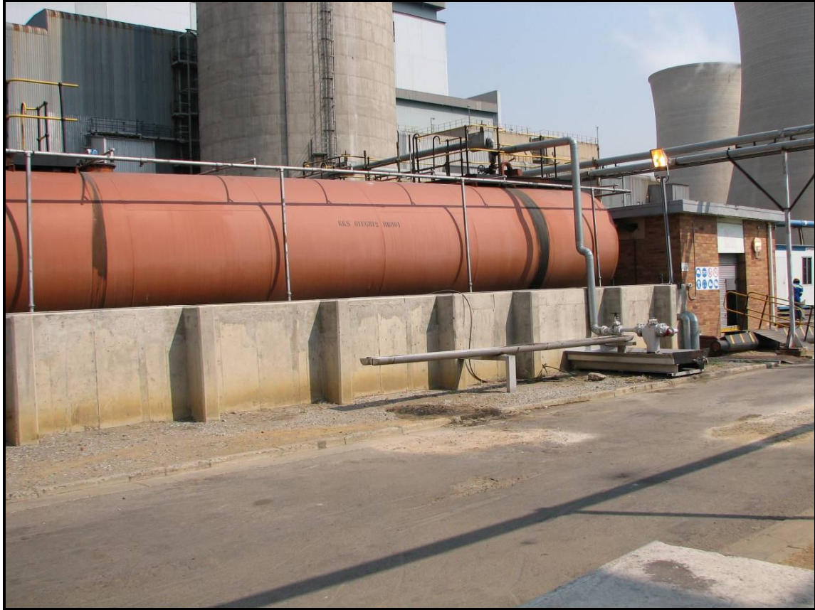
Figure 3: Photo of an existing fuel storage tank at the Grootvlei Power Station
