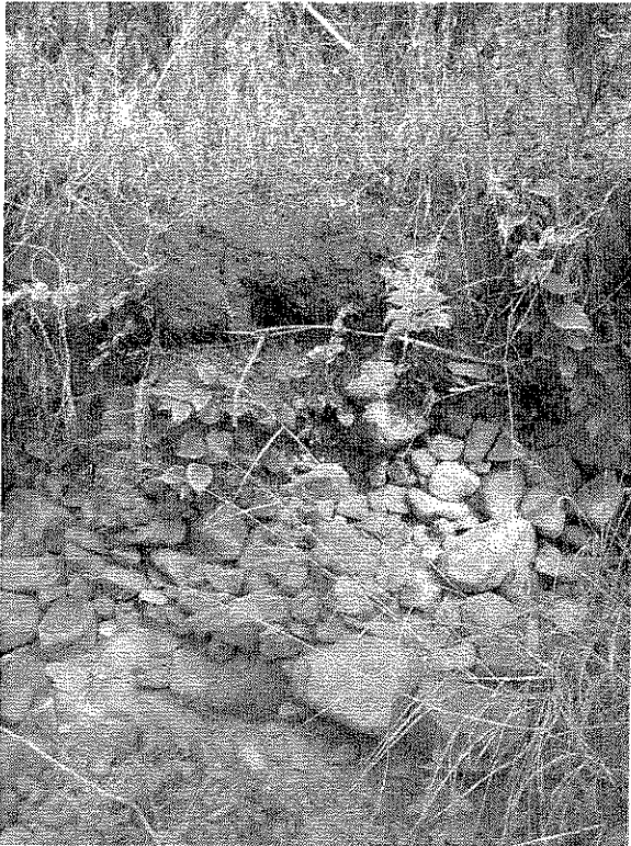
Bank Profile of the channel at appoint between LR1 and LR2. Note the shallow layer of alluvial soils overlying a pebble layer.
