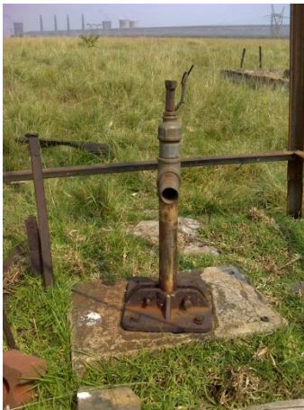
Photo 4. – Broken wind pump at FBB23.
