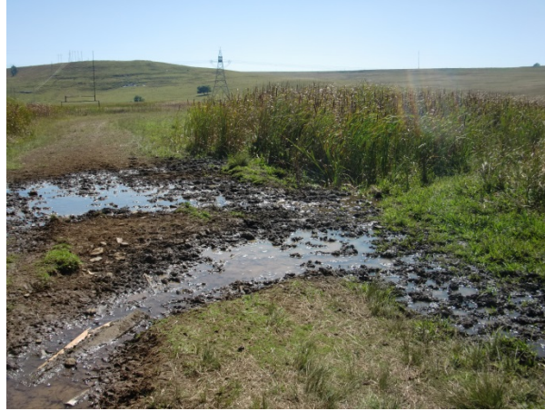
Photo 26. – Seepage at canal C26.
