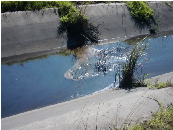
Photo 22. – Oil in canal C11.
