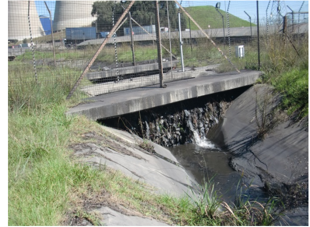
Photo 21. – Debris between the fences at canal C11.
