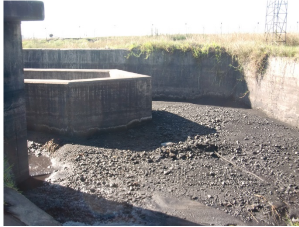
Photo 20. – Splitter box near P04.
