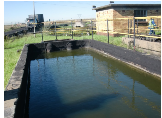
Photo 24. – Oil and silt in sump P11.
