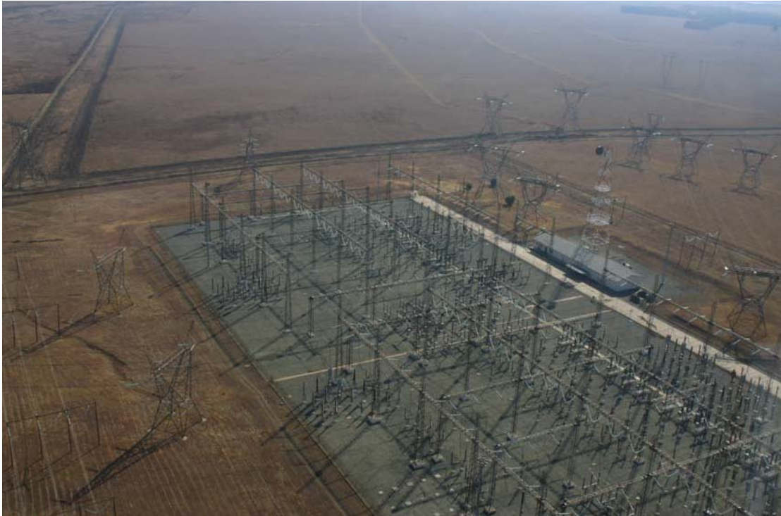
Figure Area for expansion is to the right of the existing substation as orientated this photograph
