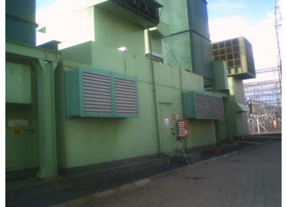
Measurements at the cooling fans
