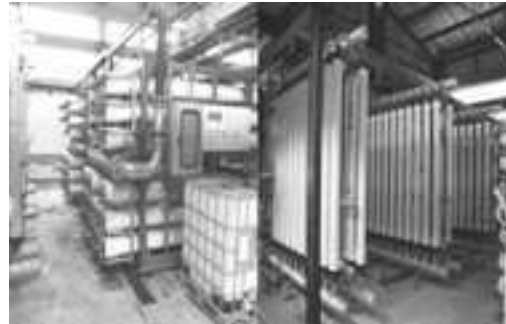
Current Spiral Wound Reverse Osmosis Plant (SRO)
