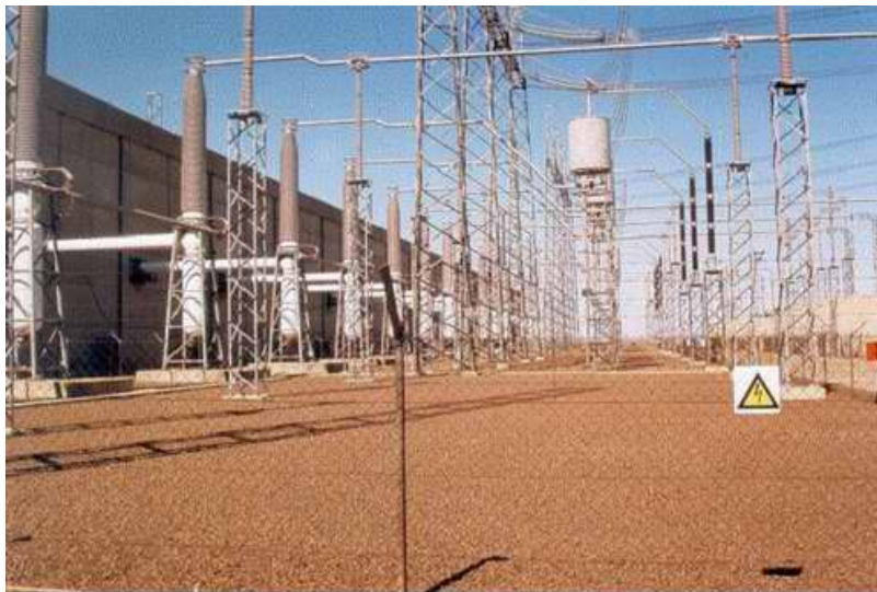
PHOTOGRAPH 16: GAS INSULATED SWITCHGEAR WITH OUTDOOR TELECOMMUNICATIONS TERMINAL EQUIPMENT
