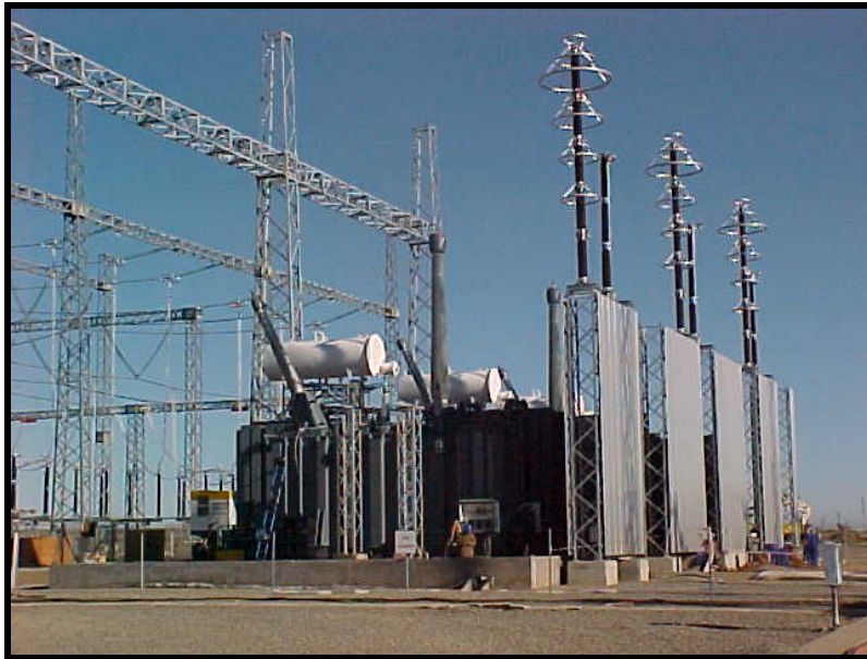
PHOTOGRAPH 15: SURGE ARRESTOR AND EARTH SWITCH MOUNTED ON TOP OF STAINLESS STEEL FIRE BARRIER, 765/400 KV TRANSFORMERS BEHIND IT AND BUSBAR STEELWORK IN THE BACKGROUND.
