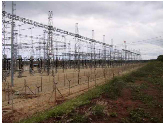
PHOTOGRAPH 17: EXAMPLE OF OVERHEAD STRUNG FLEXIBLE CONDUCTOR BUSBARS STRUCTURE
