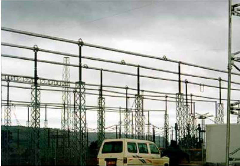
PHOTOGRAPH 5: EXAMPLE OF TUBULAR ALUMINIUM CONDUCTOR ARRANGEMENT
