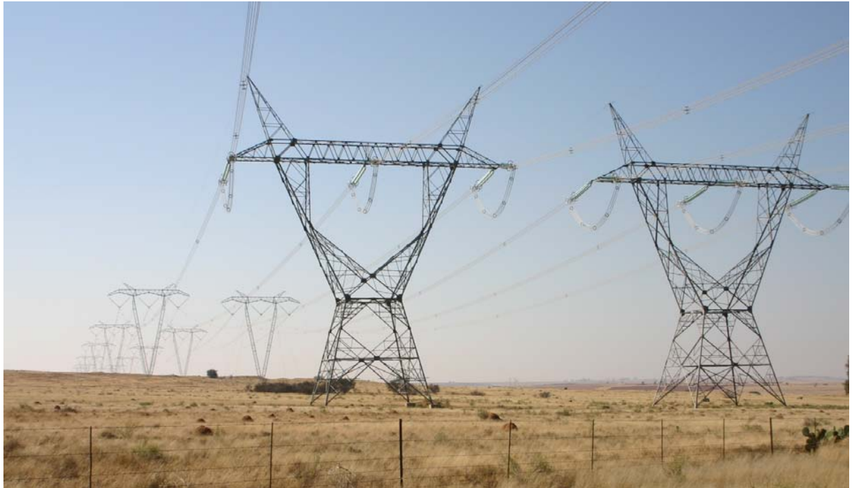
Figure 4 – Example of 765kV Strain Tower
