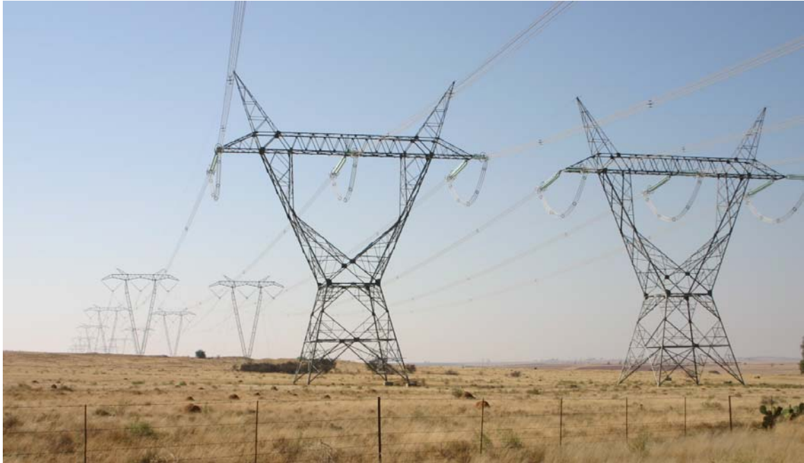
Figure 3 – Example of 765kV Strain Tower
