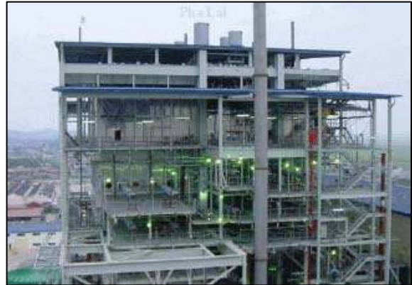
Figure 3: Typical unclad boiler
