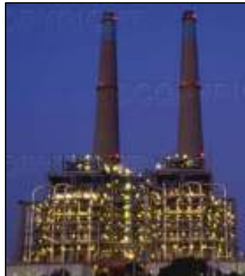
Figure 4: Typical unclad boiler at night
