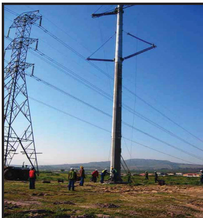
Figure 2.15: Monopole structure which can be used in areas where there are space constraints like the Magaliesberg Ridge.
