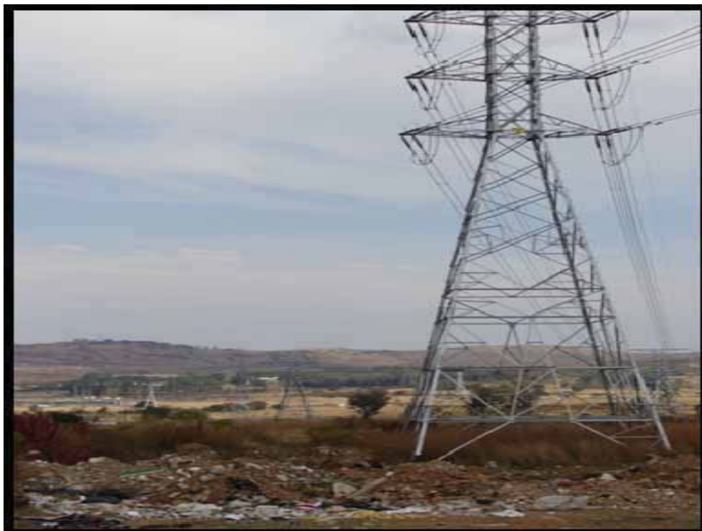
Figure 2.10: Typical self-supporting double-circuit tower used from Kwagga substation
