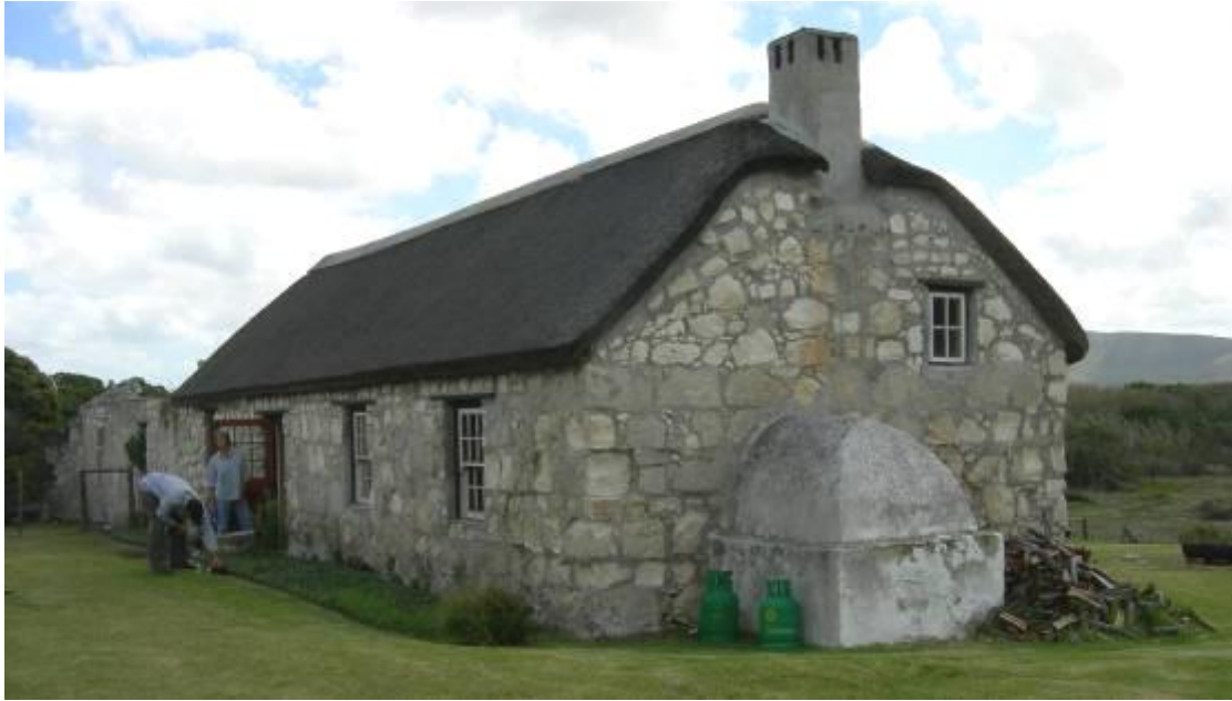
Figure 12 (above) Vernacular cottage at Groot Hagelkraal farm complex. This is a typical Cape " langhuis " built from south coast limestone. The end portion is in a ruined state.
