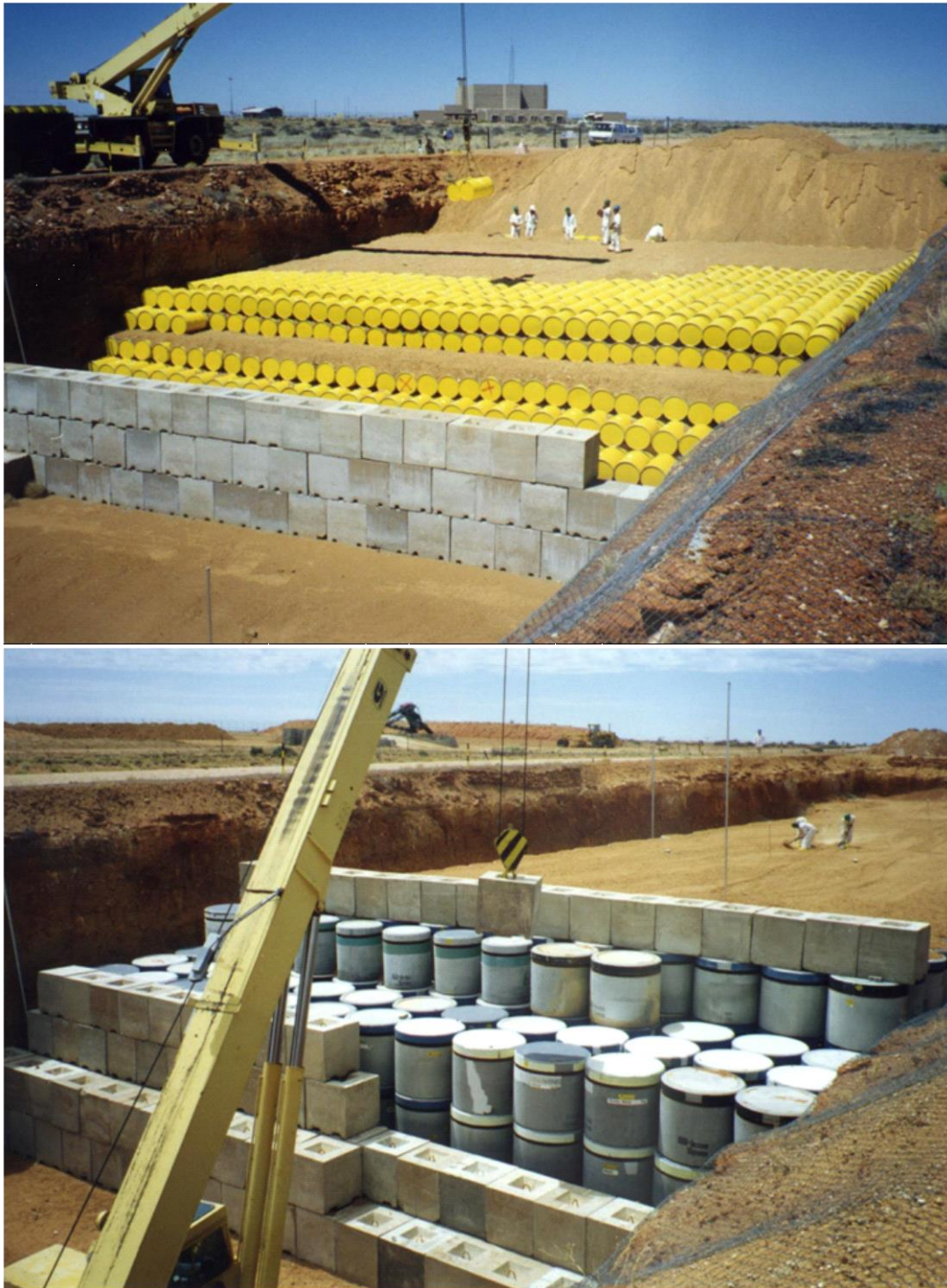
Figure 5.7: Examples of the near surface trenches used for the disposal of LLW (top) and ILW (bottom) at Vaalputs.
