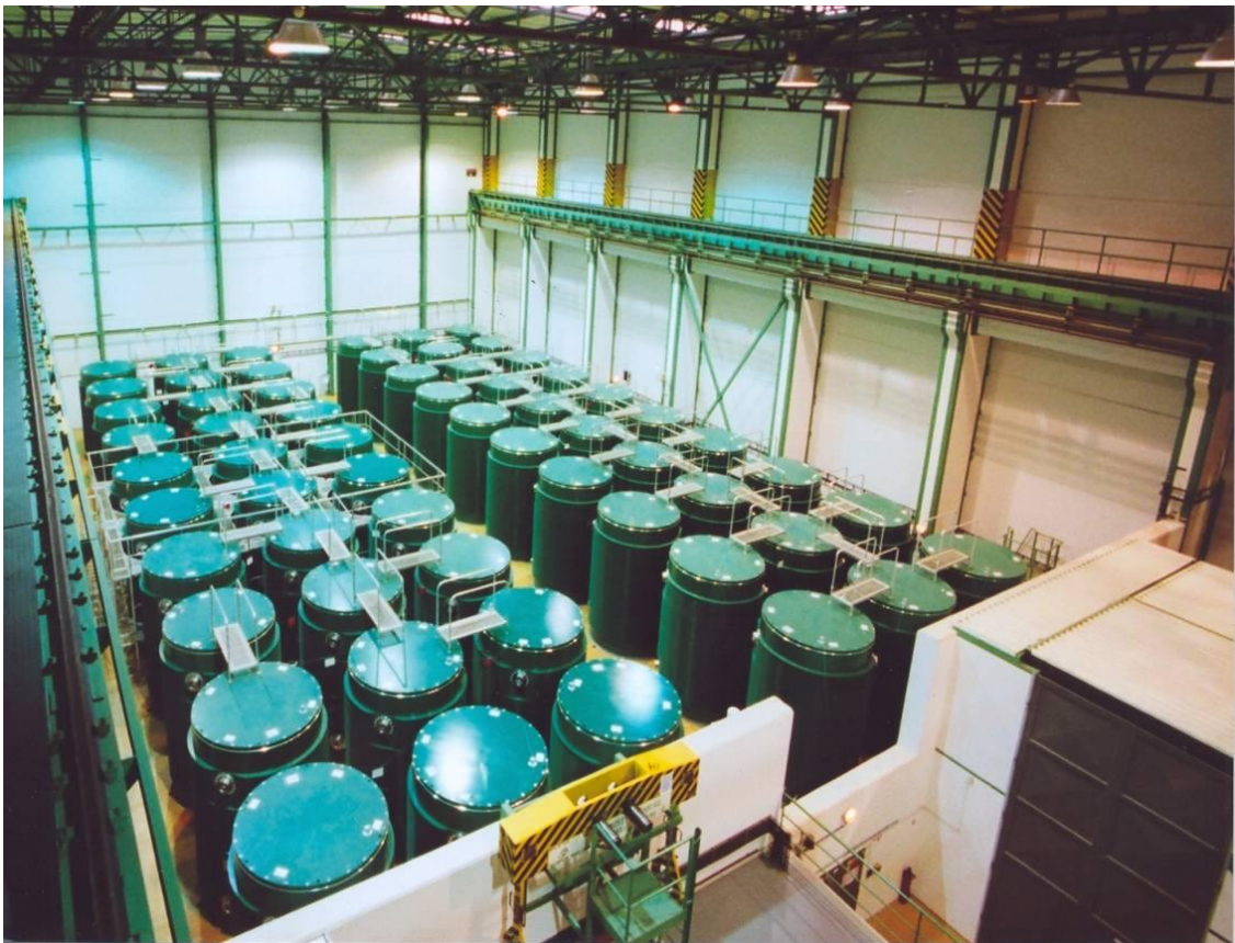
Figure 5.10: An example of a dry storage facility for spent nuclear fuel
