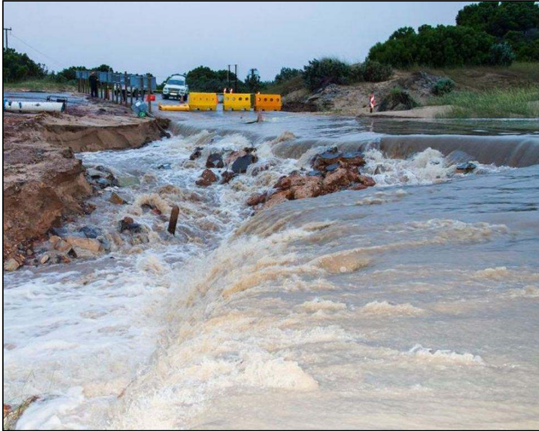
Figure 8.3 The dying moments of the Sand River culvert on 22 October 2012
