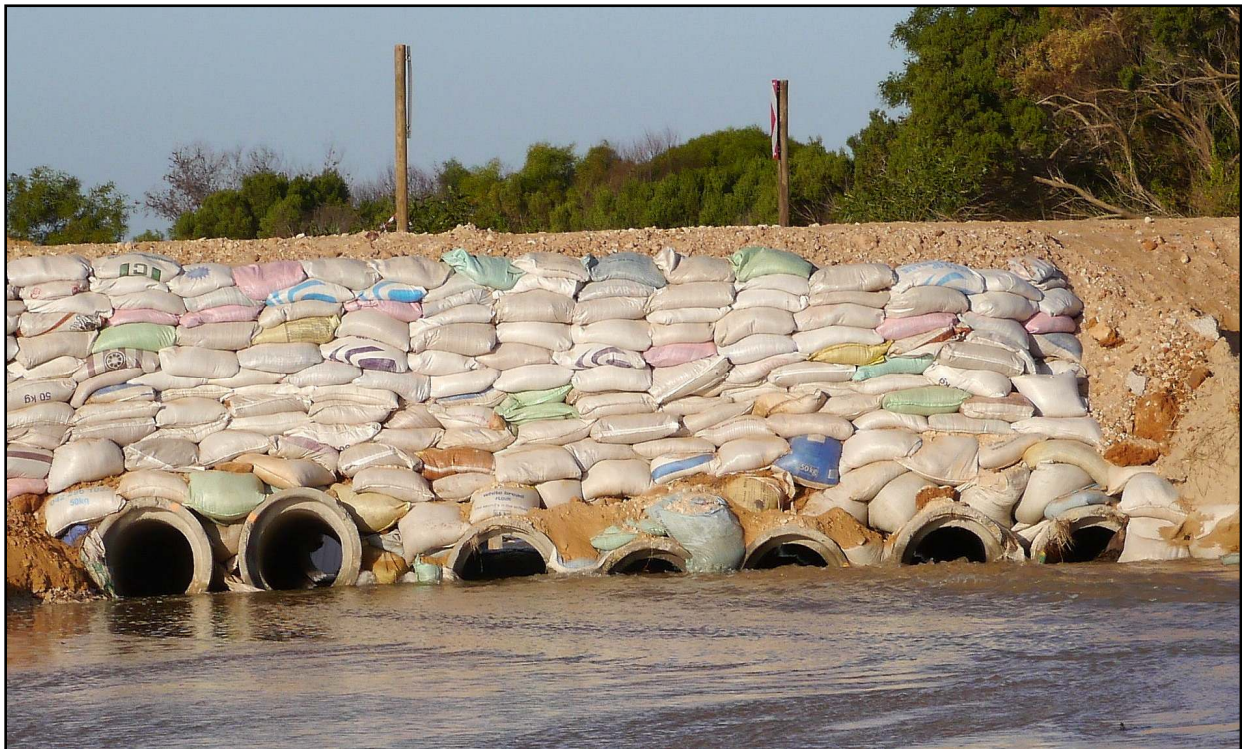
Figure 8.5 The seven pipes on the upstream side of the 2012 culvert. The pipes are not at the same level, so some of these pipes could potentially be blocked.
