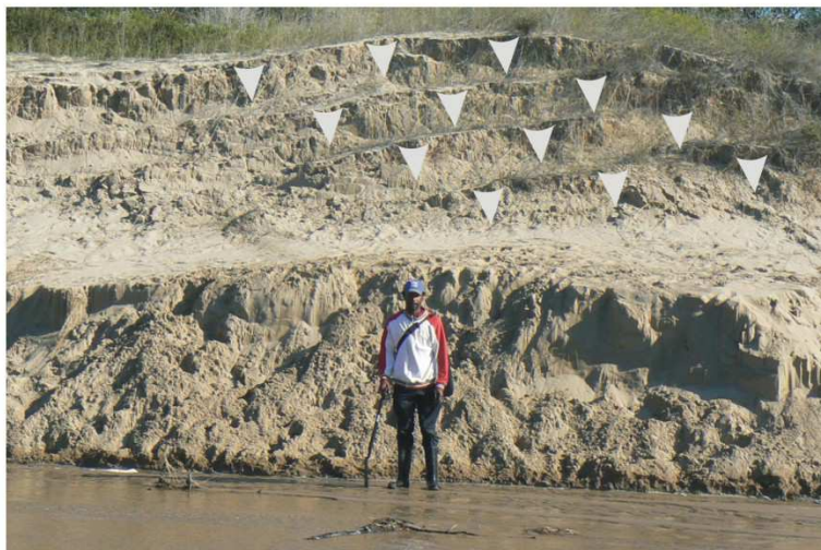
Figure 1: A series of slides (indicated by 4 sets of arrows along the slope) where slope material has moved downwards without water acting as the medium causing slope failure.
