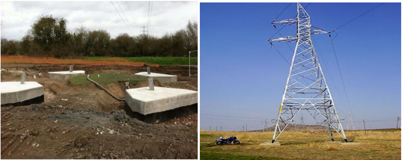
Fig 7 Showing established tower foundations with extent of disturbed area and completed tower and rehabilitate disturbed area showing grass growing at and around the tower base
