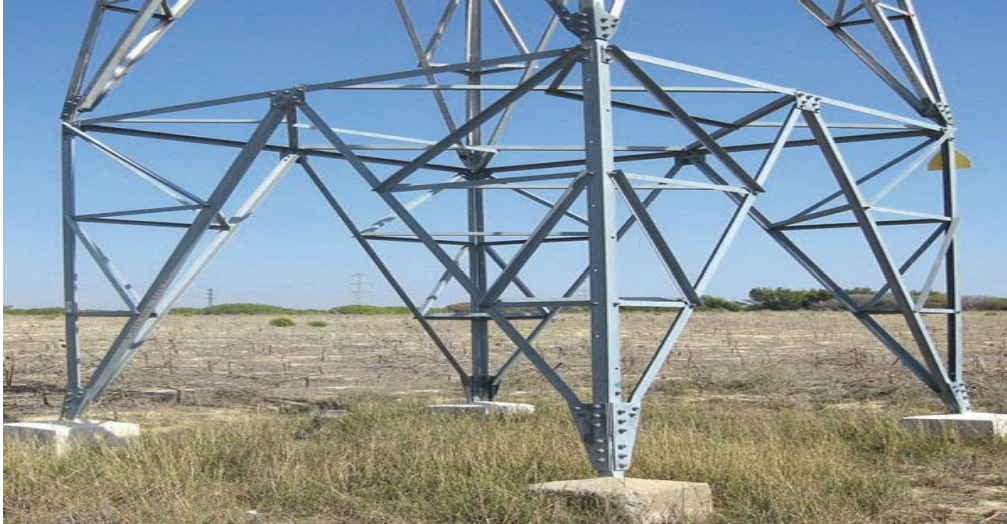
Fig 8 Showing grass growing back along tower foundation
