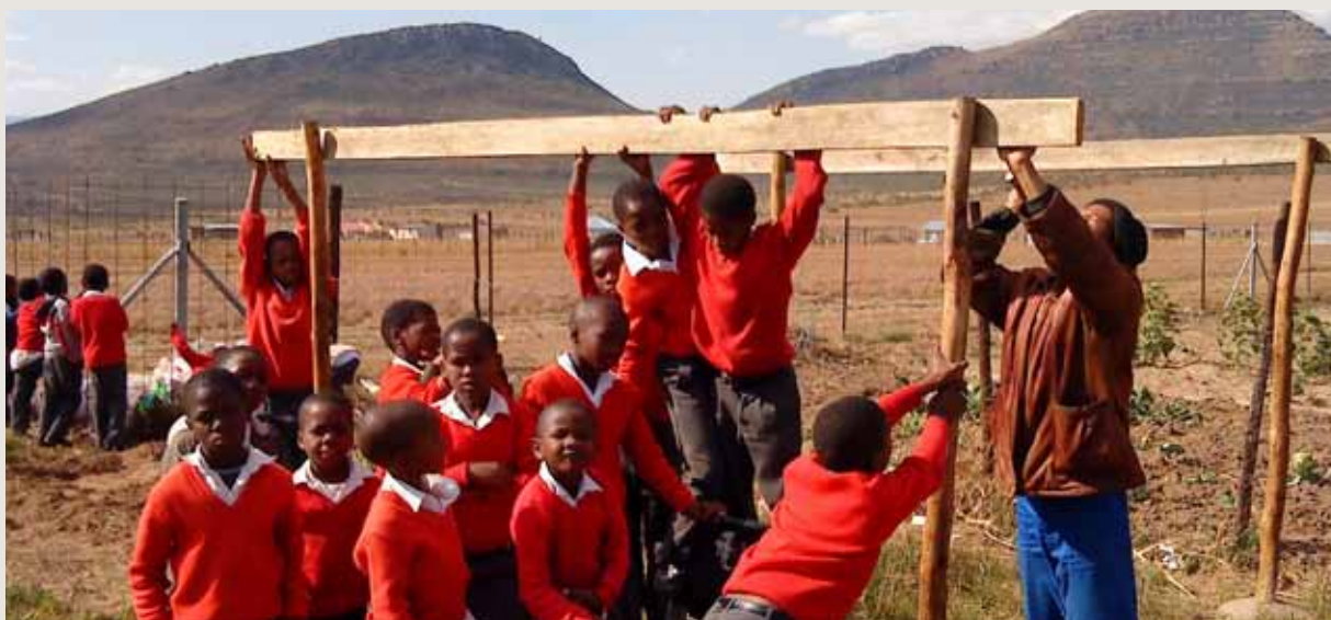
The sustainability commons at Three Crowns primary makes the leap from school to community.
