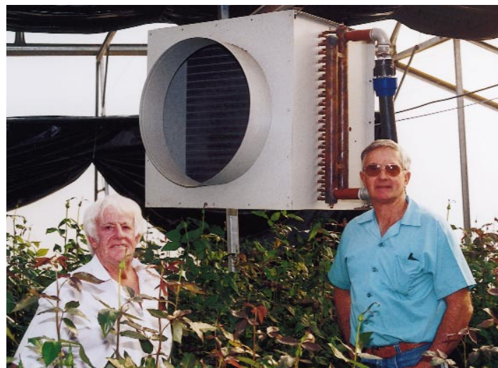
Mr Ken Gilham, Agrelek advisor (left), and Mr Peter Aitken at a heat exchanger in one of the new greenhouses.
