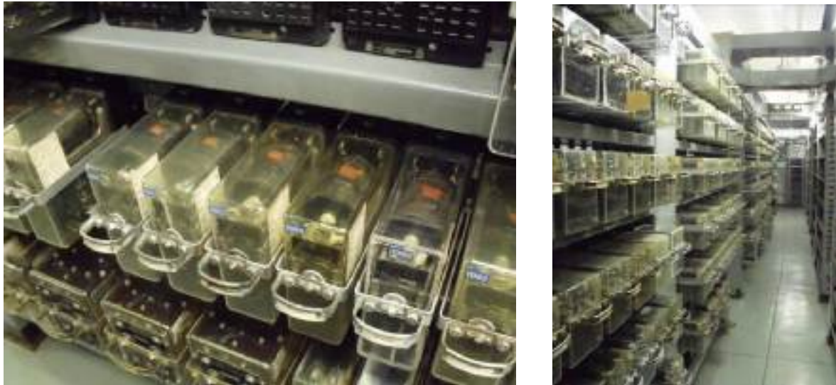
Figure 3-5: Example of the contents of a relay room.
