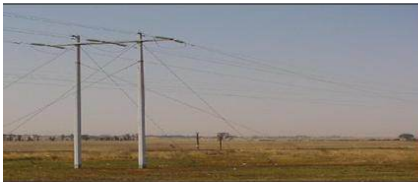
Figure 3-8: Example of a low voltage distribution power line.
