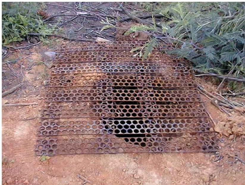
Photograph 2.1: Prior to filling of the foundations and tower erection, excavated foundations are covered in order to safe-guard unsuspecting animals and people from injury
