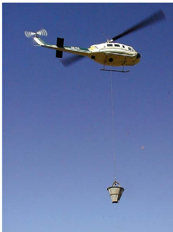
Photograph 2.2: In the event of the site being inaccessible, concrete is delivered to the site by helicopters
