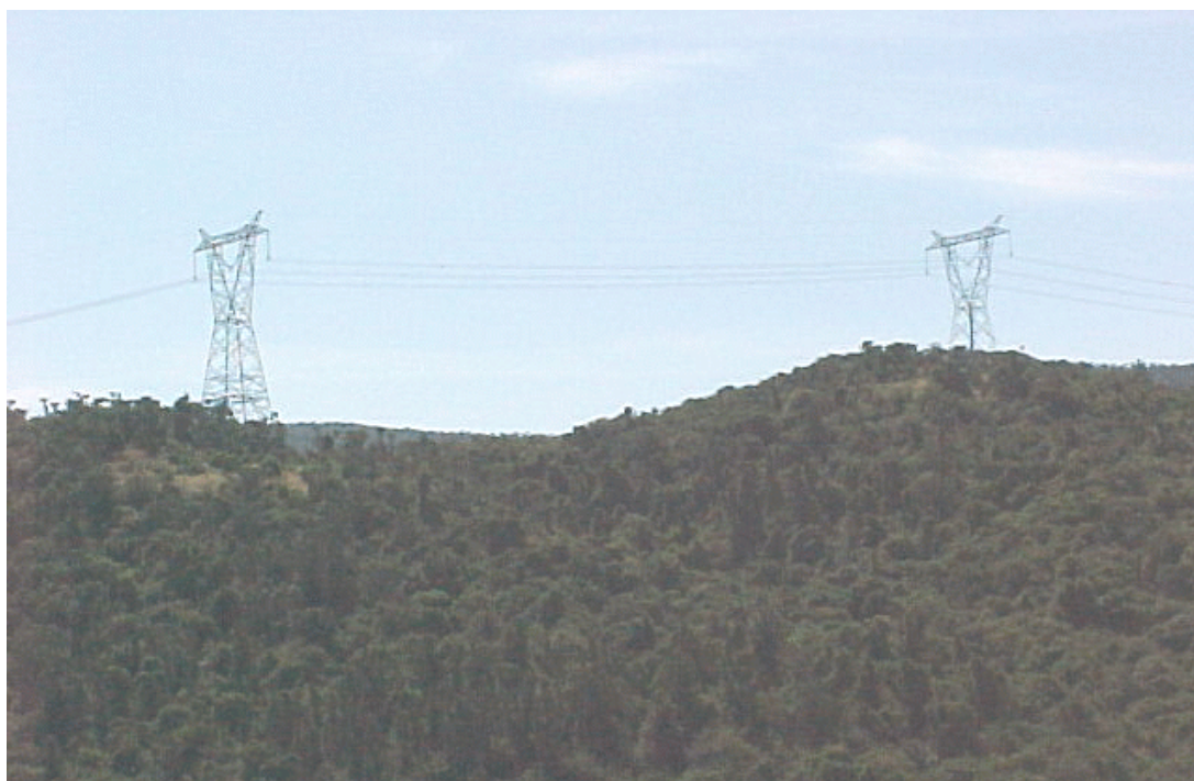
Photograph 10.2: The existing 220 kV Transmission lines over the Zuurberg mountains have a high visual impact where towers are exposed against the skyline. Such placement of towers should ideally be avoided.
