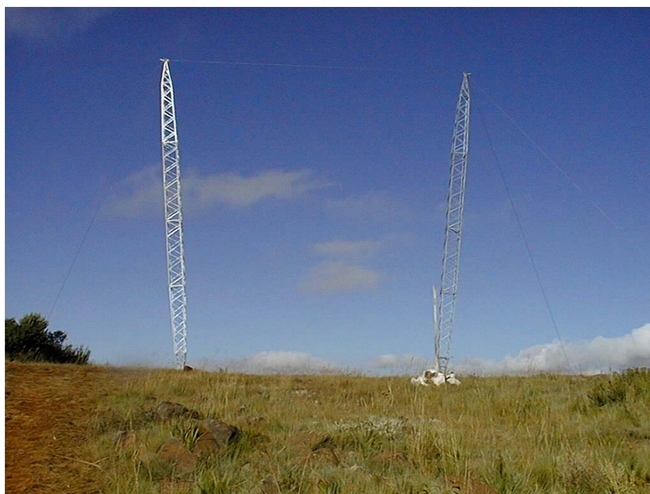
Photograph 10.3: The proposed Transmission line will be constructed using CRS towers which are smaller, less steel-intensive, and less visually intrusive than those towers of the existing Transmission lines
