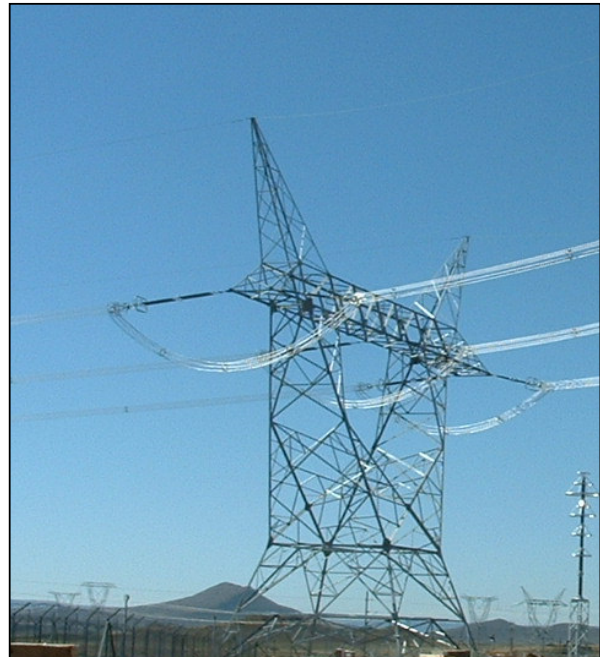
Self-supporting 765kV Strain Tower
