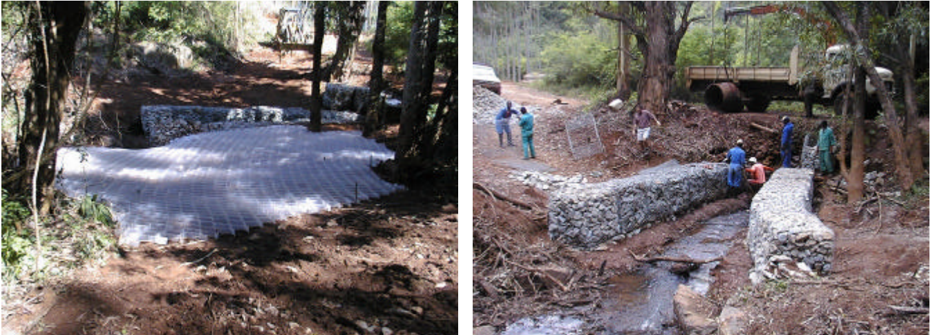
Figure 3. Extensive measures taken to prevent erosion, during the construction of access roads for a new power line. Continuous cellular mat (left) and gabions (right) are some of the measures used during the building of access roads during the construction phase of a power line. (Photos: Jose Clara).
