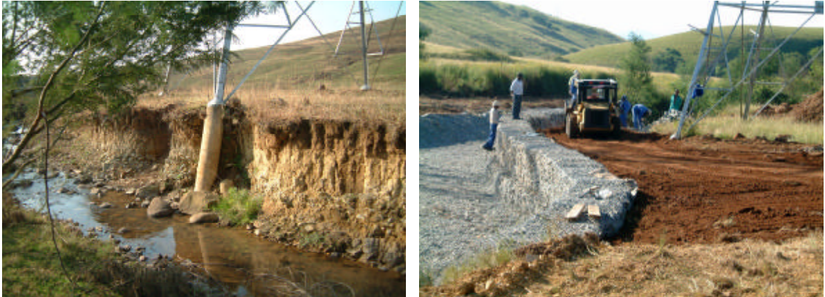
Figure 1: The photo on the left shows the foundation of a tower exposed by erosion. The photo on the right shows the extensive and costly remediation by using gabions and reno mattresses. Also note the use of good topsoil that will permit the re-establishment of vegetation around the tower (photos Jorge Correia).
