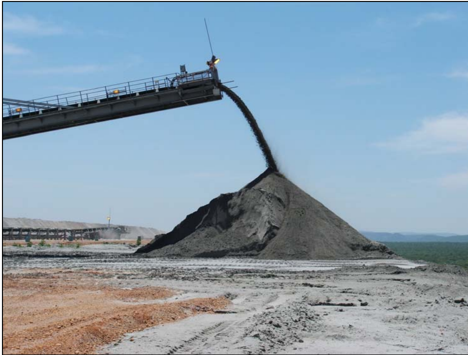
Figure 9.13: Stacking of ash by stacker at the Zwartwater ash dump. The relatively high moisture content of the ash reduces the potential for fugitive emissions during this process.
