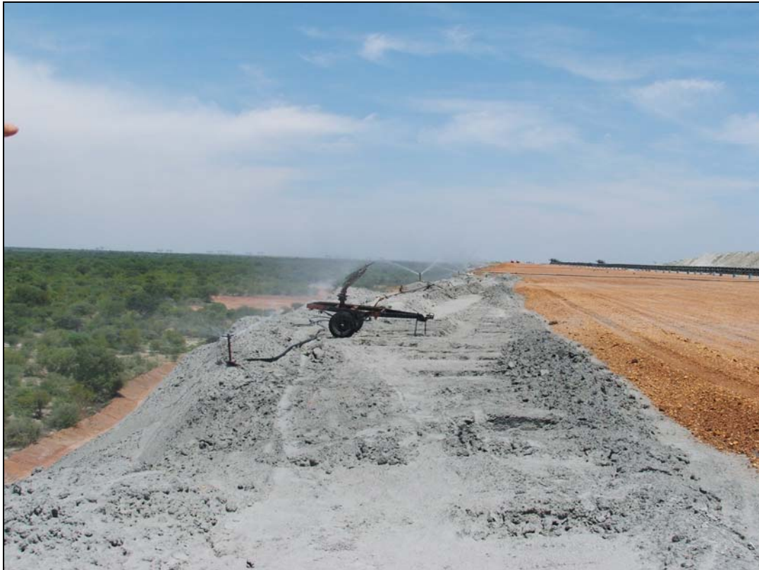
Figure 9.11: Southern side of the ash dump at Zwartwater, with the topsoil covering of the ash and the use of wet suppression evident.
