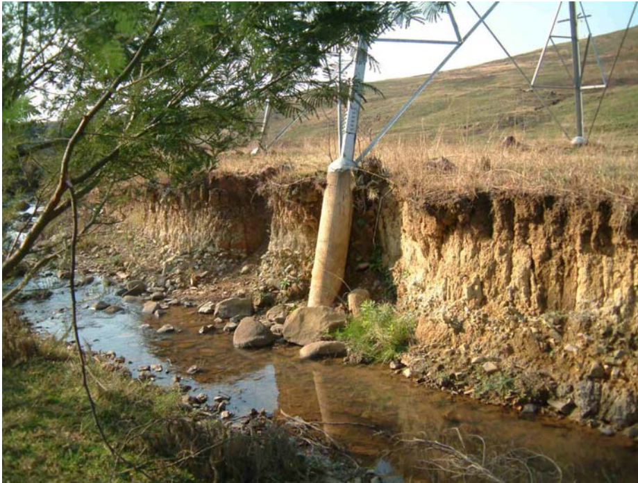
Figure 8. Example of the dangers of erosion to power lines (photo Jorge Correia).
