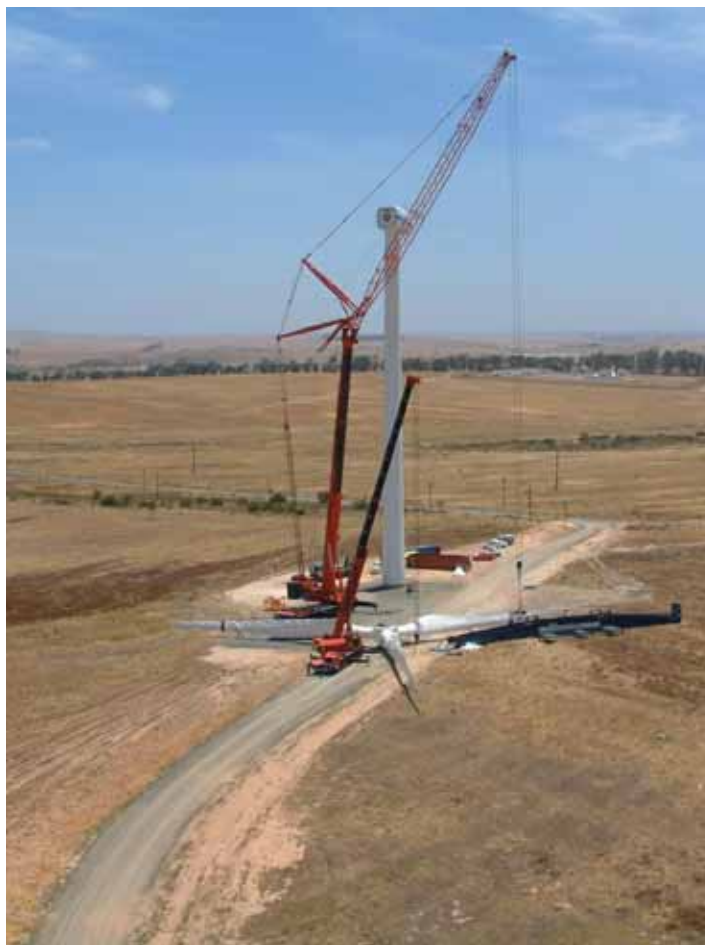
Figure 5.4: Photograph illustrating the laydown areas required during the erection of one of the turbines at the Klipheuwel demonstration facility (photo courtesy of Eskom)
