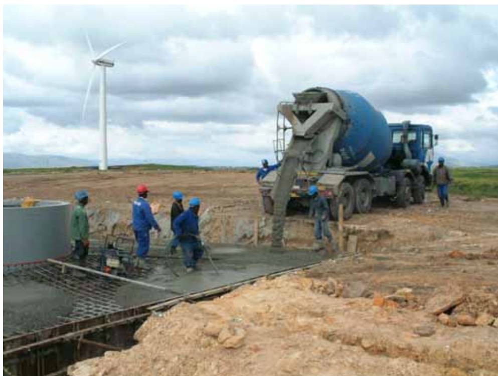
Figure 5.5: Photograph illustrating the construction of the foundation of one of the turbines at the Klipheuvel demonstration facility (photo courtesy of Eskom)
