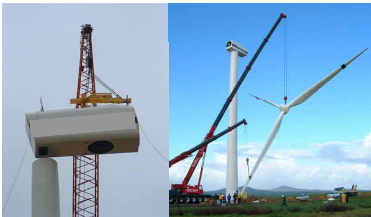
Figure 5.8: Photograph illustrating the assembly of a turbine (nacelle and blades) utilising a large lifting crane (photographs courtesy of Eskom from construction at the Klipheuwel demonstration facility)
