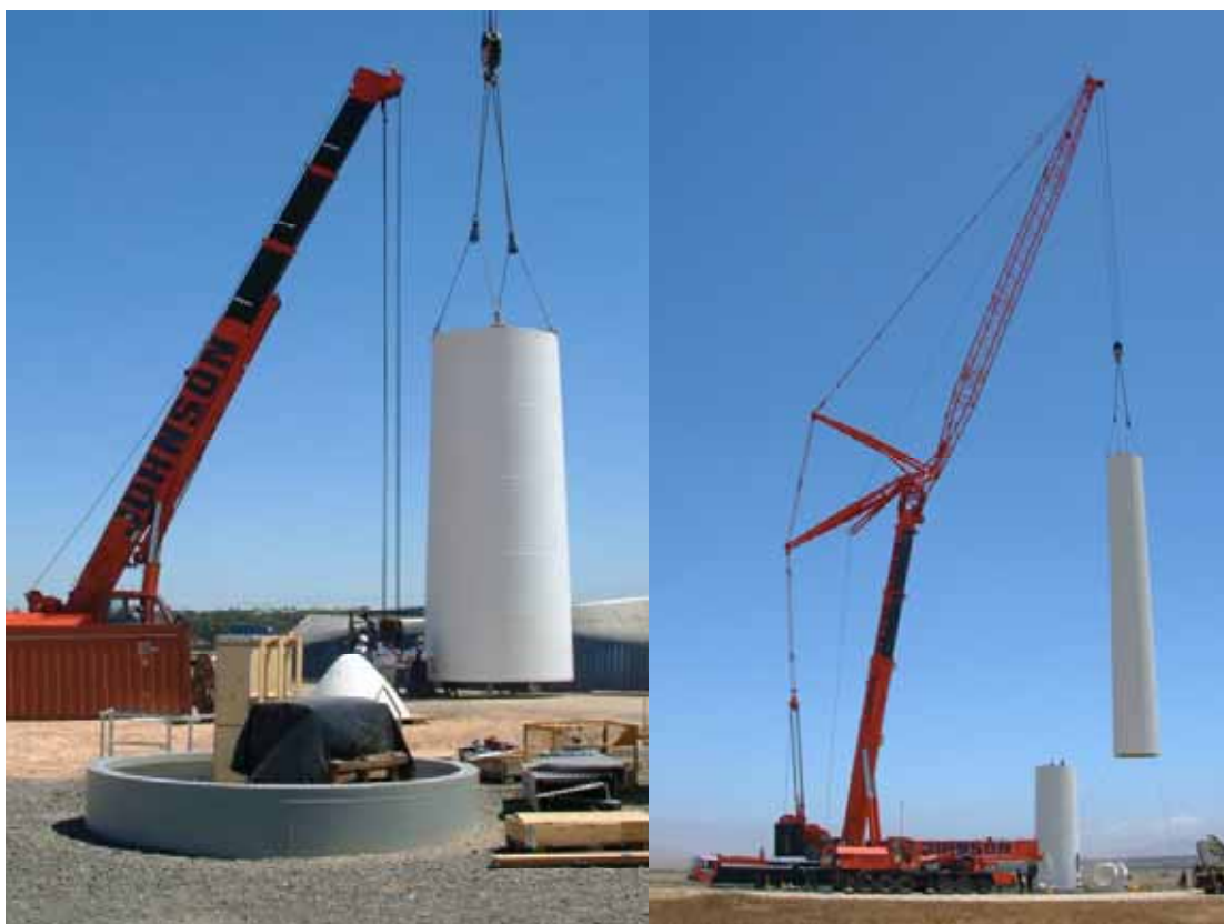
Figure 5.7: Photograph illustrating the assembly of a turbine tower utilising a large lifting crane (photographs courtesy of Eskom taken during the construction of the Klipheuwel demonstration facility)
