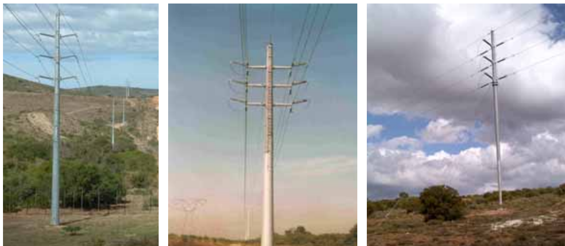
FIGURE 8. Double-circuit mono-pole pylon designs favoured to carry the Juno-WEF 132 kV power line: intermediate structure (left), standard strain (centre) and stayed strain (right), all with guard wires fitted.
