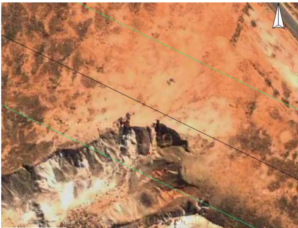
Figure 16. Scarp likely to be associated with slope failure and a high erosion risk. The headcut is expected to migrate further upslope and hence will pose a threat to any tower located in this area.
