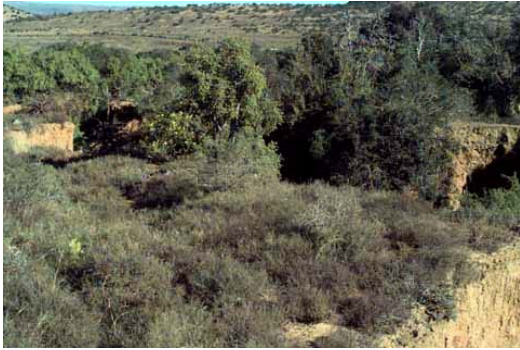
Figure 20. Deep alluvial soils are eroded by road or human activities and this is a high risk when building access roads. Jointed cactus is a potential threat and should be monitored.
