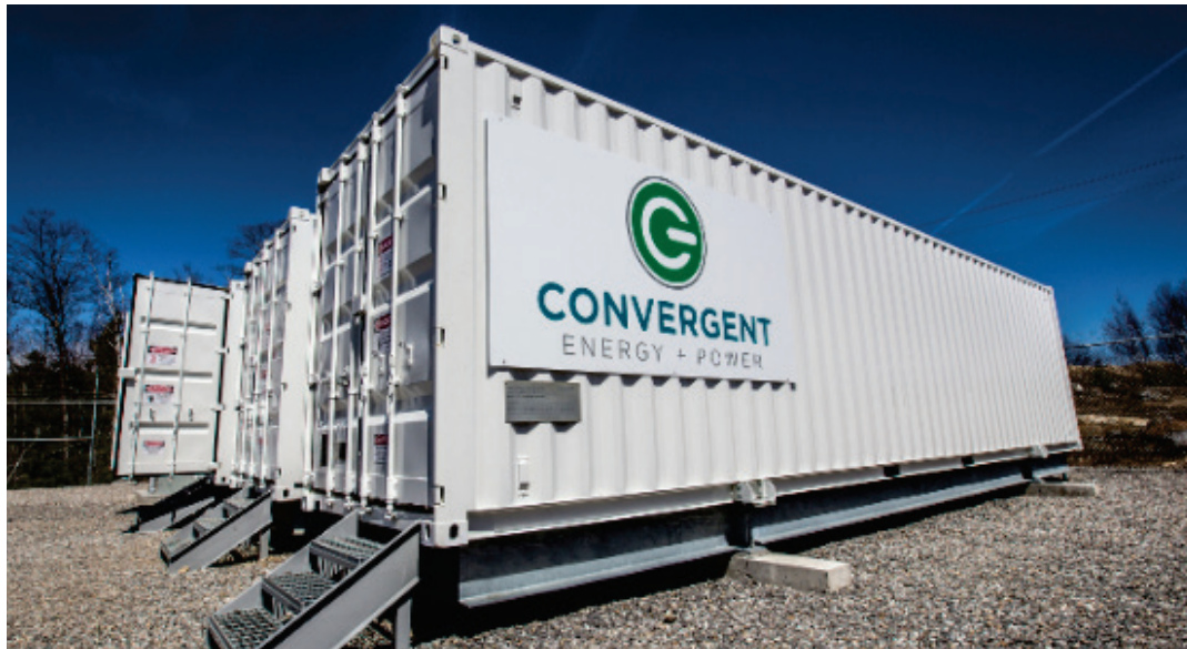
Lockheed Martin 500-kW/3-MWh energy storage system in Boothbay, Maine.
