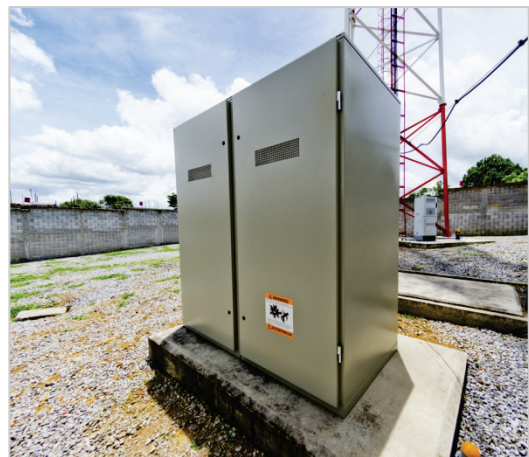
Fluidic Energy DC Energy Storage System
