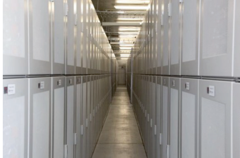
Inside the Tehachapi Energy Storage project.
