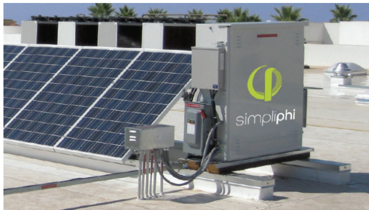
Example: SimpliPhi systems providing renewable energy integration.
