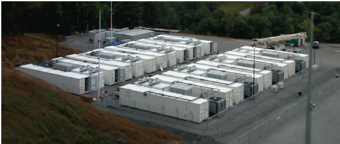
An NEC 32-MW/8-MWh GSS grid energy storage solution provides frequency regulation in Laurel Mountain, West Virginia.
