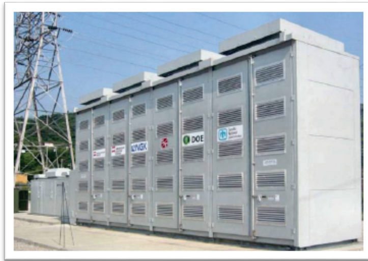
1-MW / 7.2-MWh sodium-sulfur BESS at substation for T&D deferral
