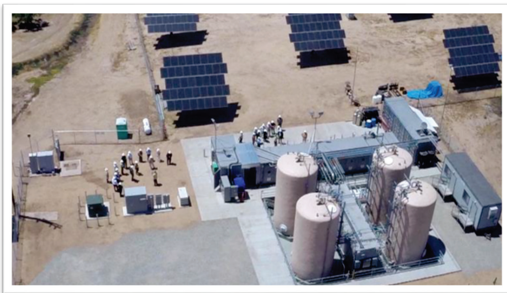
EnerVault 250kW/1MWh Iron-Chromium Flow Battery System
