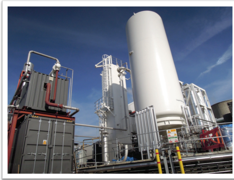
350-kW/2.5-MWh LAES Pilot Plant (courtesy Highview Power)
