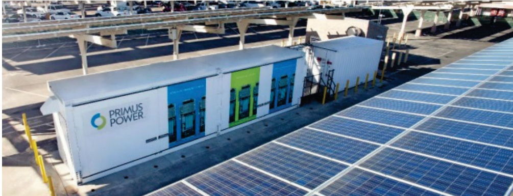
Primus Power 280-kW/1-MWh EnergyPod system installed at Miramar Marine Corps Air Station.
