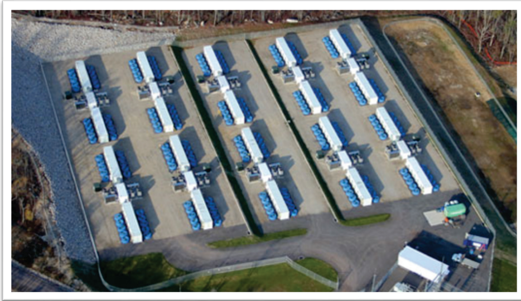
20-MW (15-minute) flywheel energy storage facility (courtesy Beacon Power)
