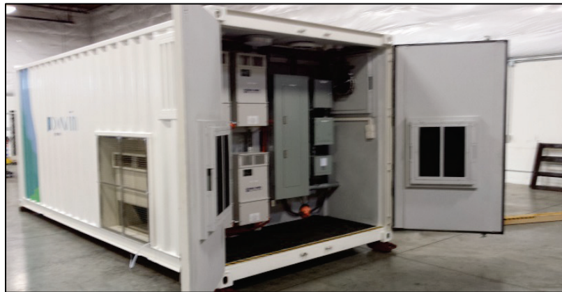
Powin Li-ion BESS in 20-ft container.
