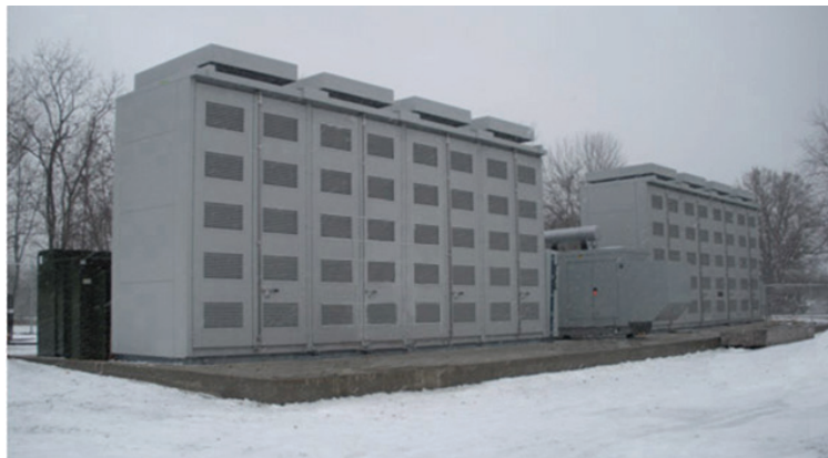
S&C 2 MW SMS provides for Islanding.
