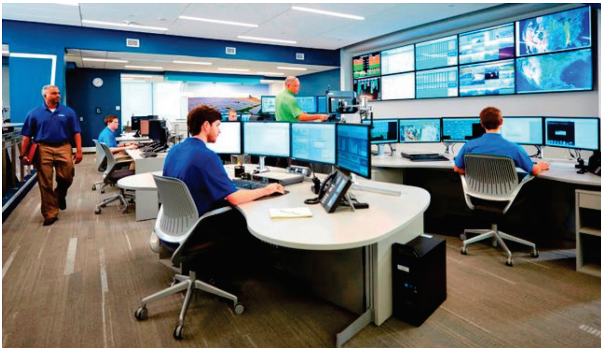
Figure 3-3: Duke Energy Renewable Control Center in Charlotte NC
