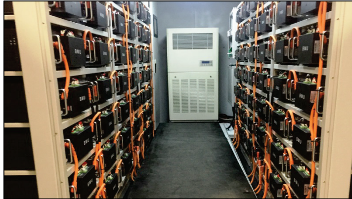
Battery racks inside a Powin containerized BESS.
