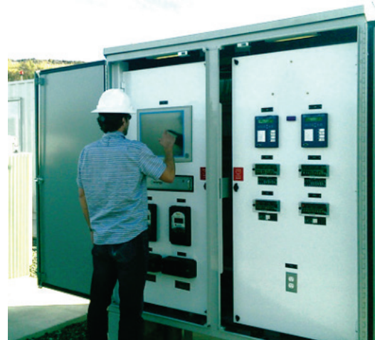
Field-deployed 1Energy 1E-IC system.
