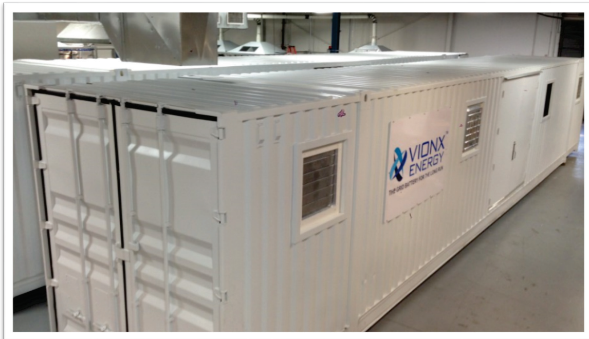
Vionx's Pilot VRB containerized energy storage system at Ft. Devens, Massachusetts
