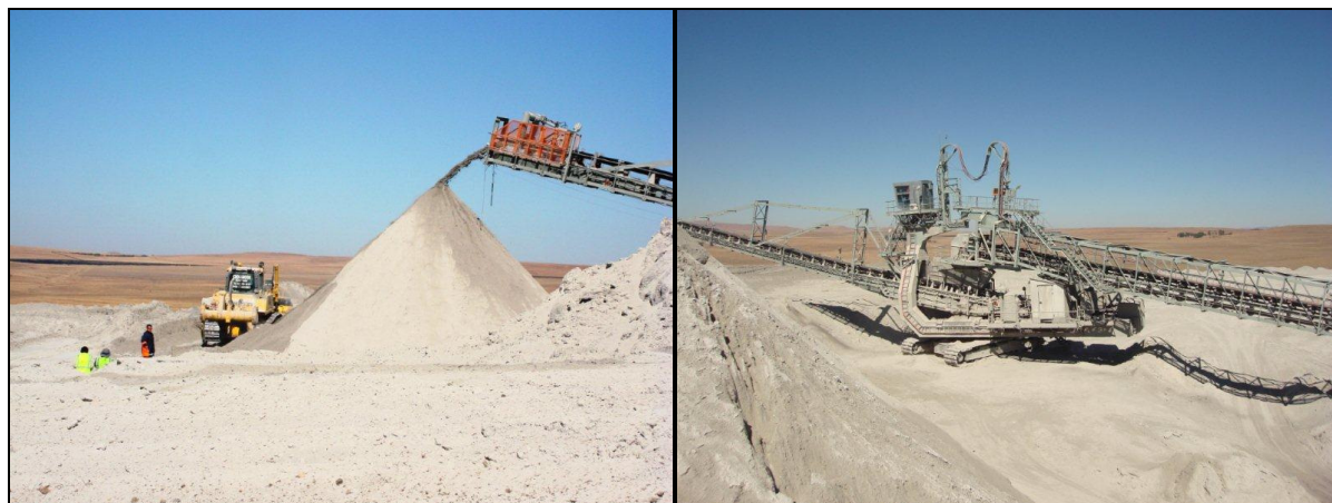
Figure 10.1: Stacker being used to dispose of ash at the Majuba power station
