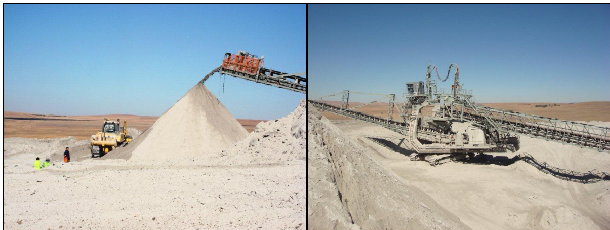
Figure 4.4: Stacker being used to dispose of ash at the Majuba Power Station
