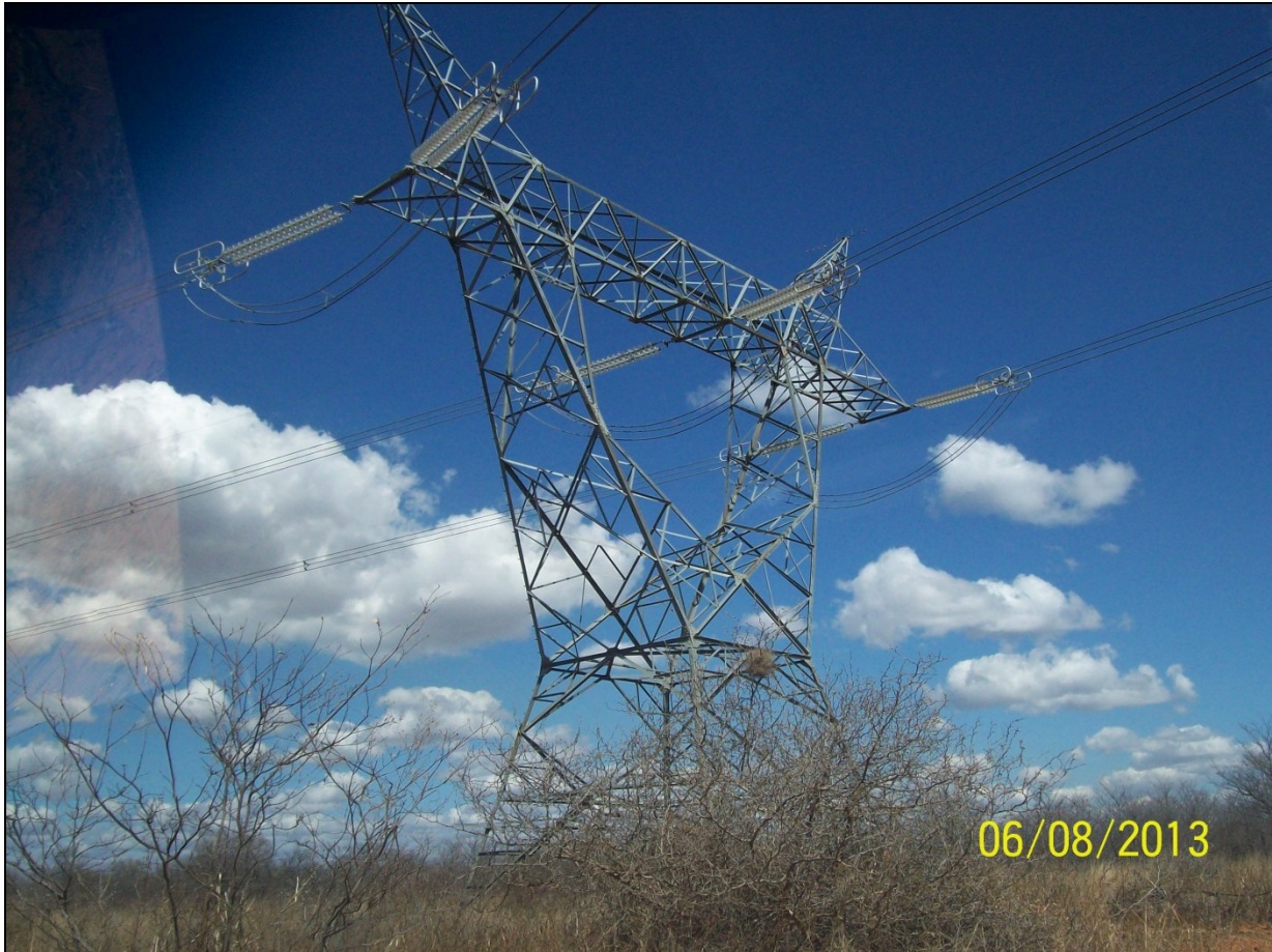
Figure 35: Eskom power line traversing site alternative two
