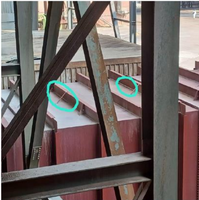
Figure 4: Duct Box Roof – Weld Fatigue
