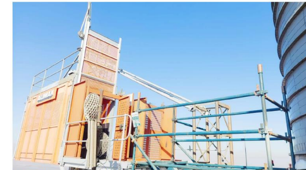
Figure 7: Alimak – Roof access and additional mast bracing
