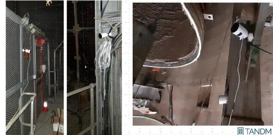
Figure 7: 55m, 151m & 180m Platforms – Cameras Installed to Visually Monitor Equipment
