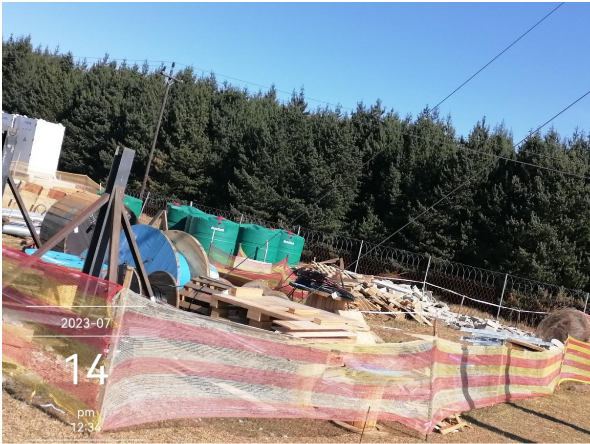
Figure 7: No go areas properly demarcated
