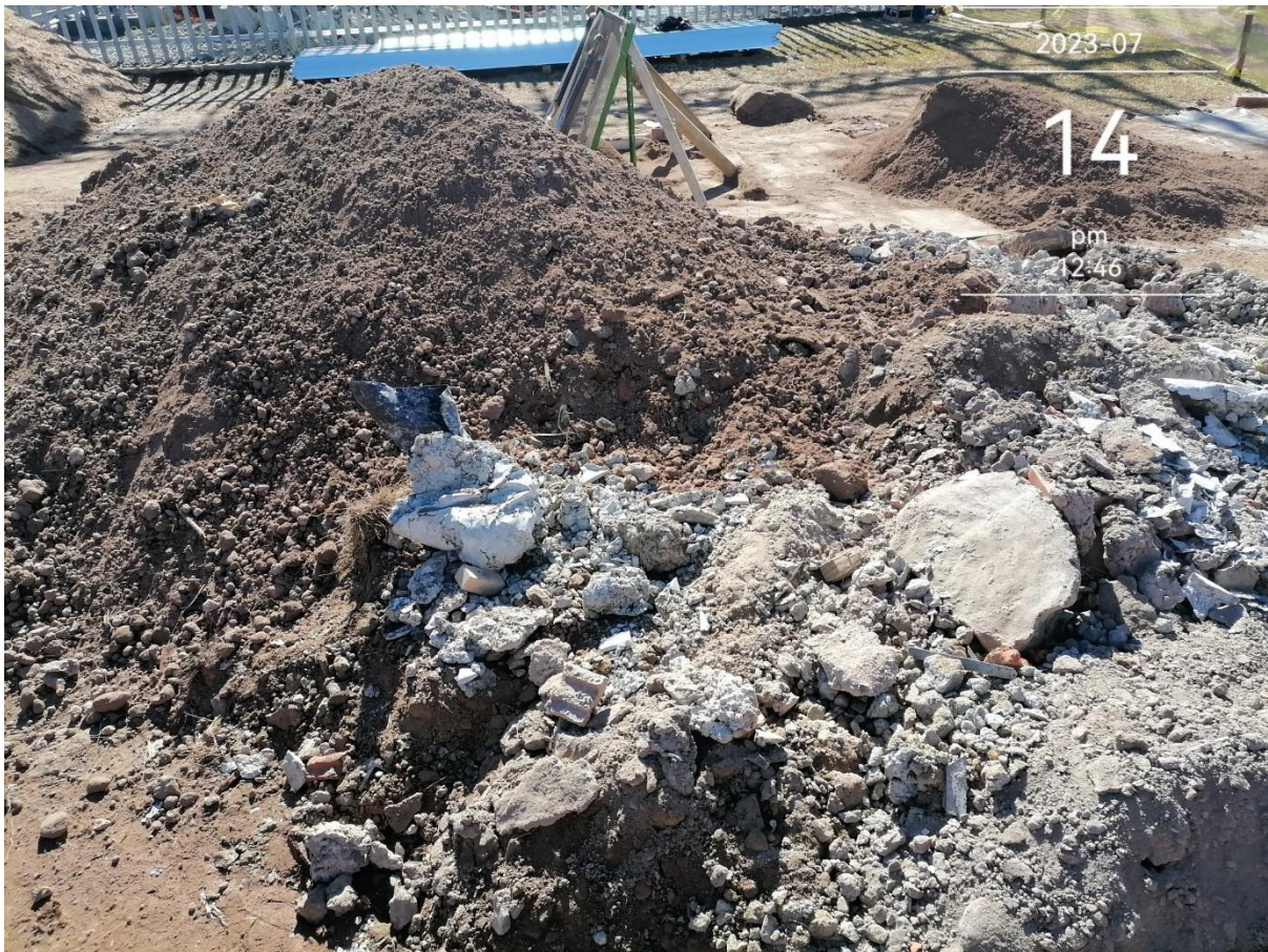
Figure 1: Building rubble not separated and not inside Skips posing soil contamination risk
