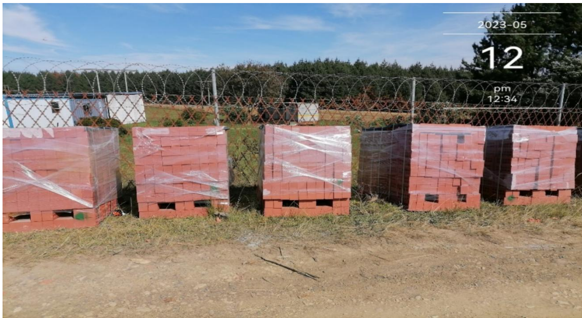
Figure 9: Shows bricks delivered outside the precinct of the Elandskop Substation
