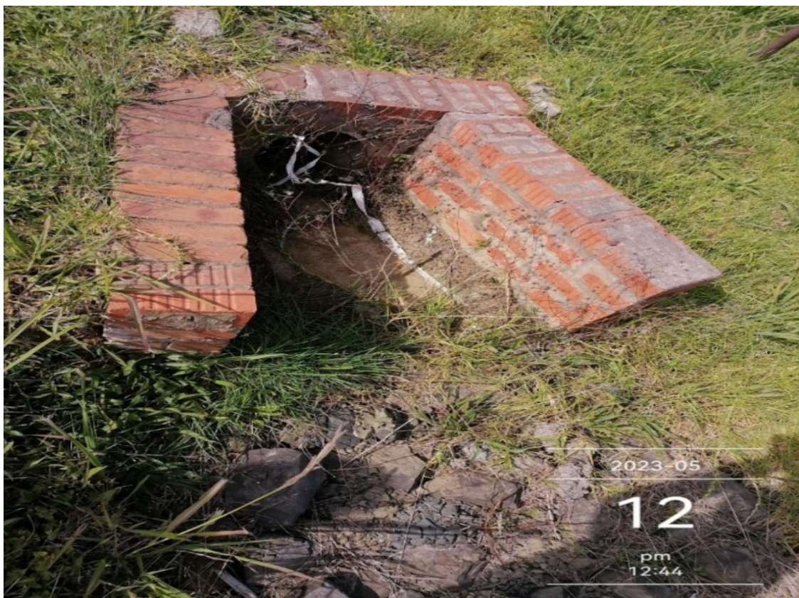
Figure 10: Evidence of storm water drainage kept clean and clear of blockage material
