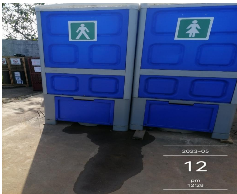
Figure 1: Toilet leak observed to be further investigated if its water or worse
