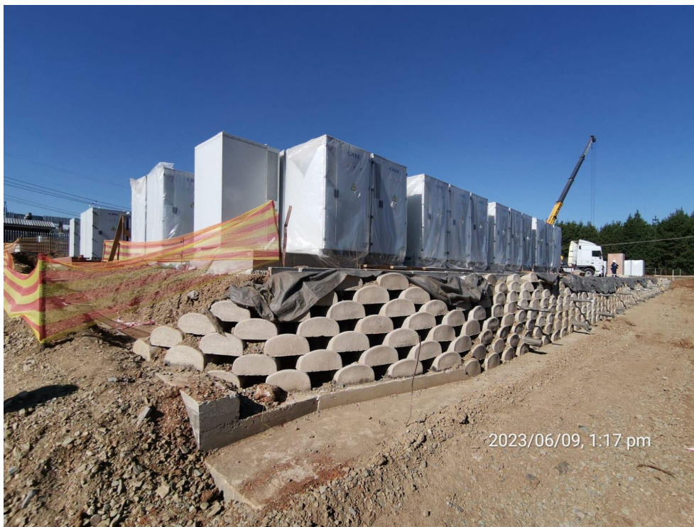
Figure 9: Soil erosion measures using curbing bricks evident
