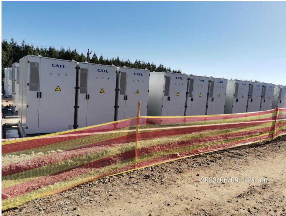
Figure 8: No go areas properly demarcated
