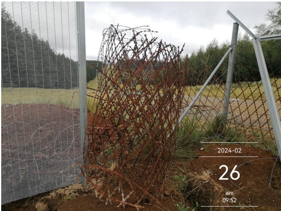
Figure 2: Scrap Fence to be disposed off properly
