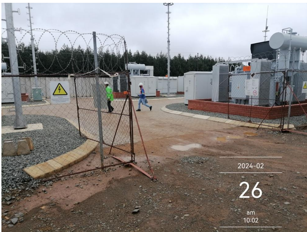
Figure 8: BESS area has no entrance gate as yet
