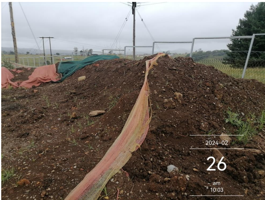
Figure 6: Top soil totally exposed not covered at all
