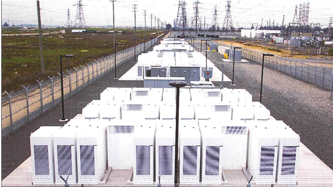
Figure 2: Lithium-ion Power Pack Units
