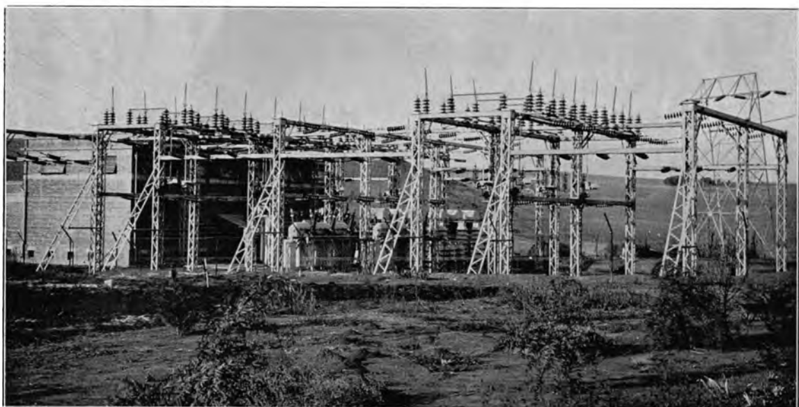
New Leigh Sub-Station.
