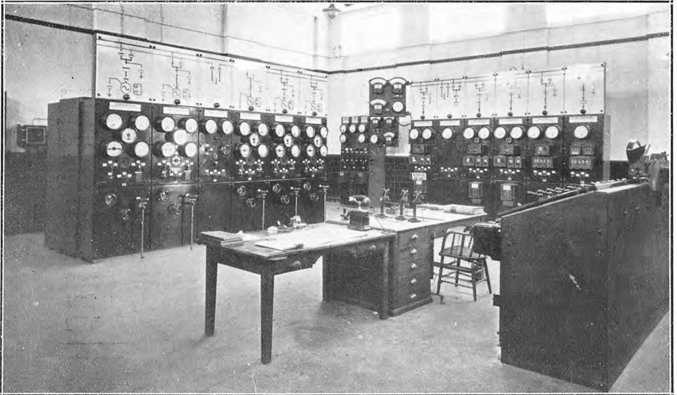
Natal Central Undertaking—Colenso Power Station: Control Room.
