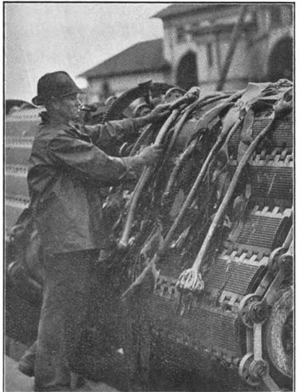
Bottom Right: Portion of Seaweed removed from the Intake Pits and Screens.
