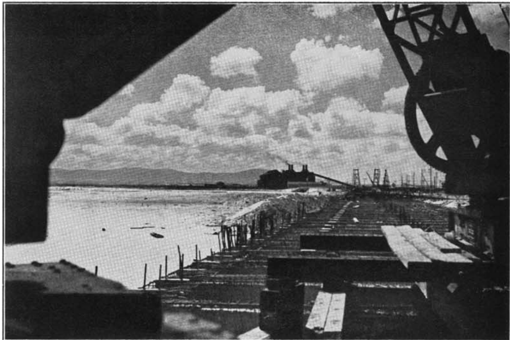
New Circulating Water Intake. View looking towards the Salt River Power Station.
