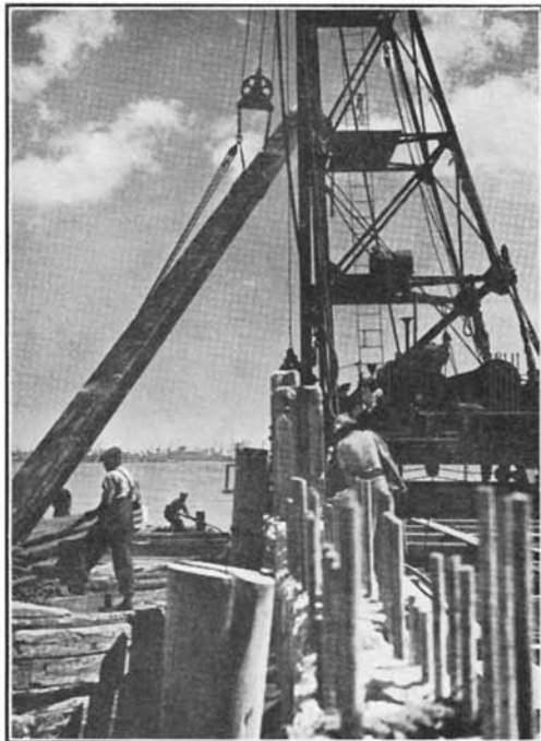
Construction of new Circulating Water Intake, Salt River Power Station. Pile-driver at work in Table Bay.
