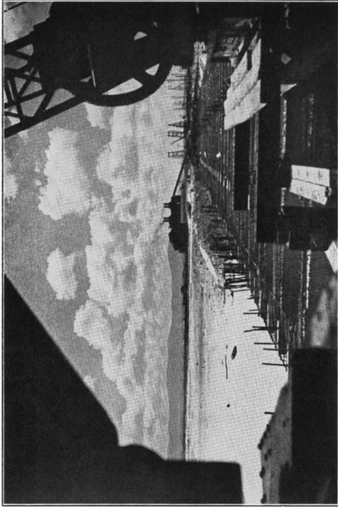
New Circulating Water Intake. View looking towards the Salt River Power Station.
