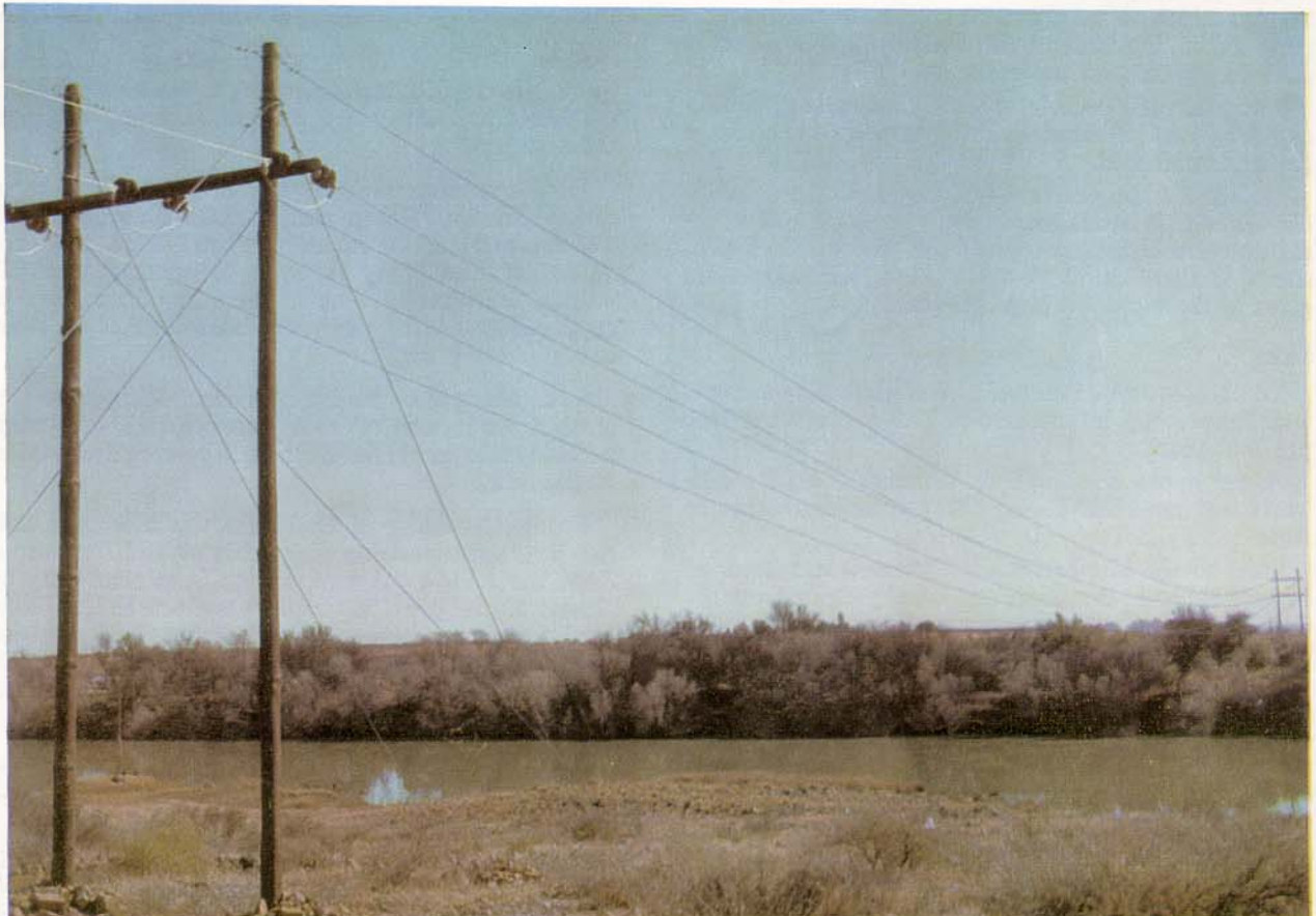
An 11 kV wood-pole transmission line crossing the Vaal River. The line forms part of a farm scheme in the Cape Northern Undertaking.
