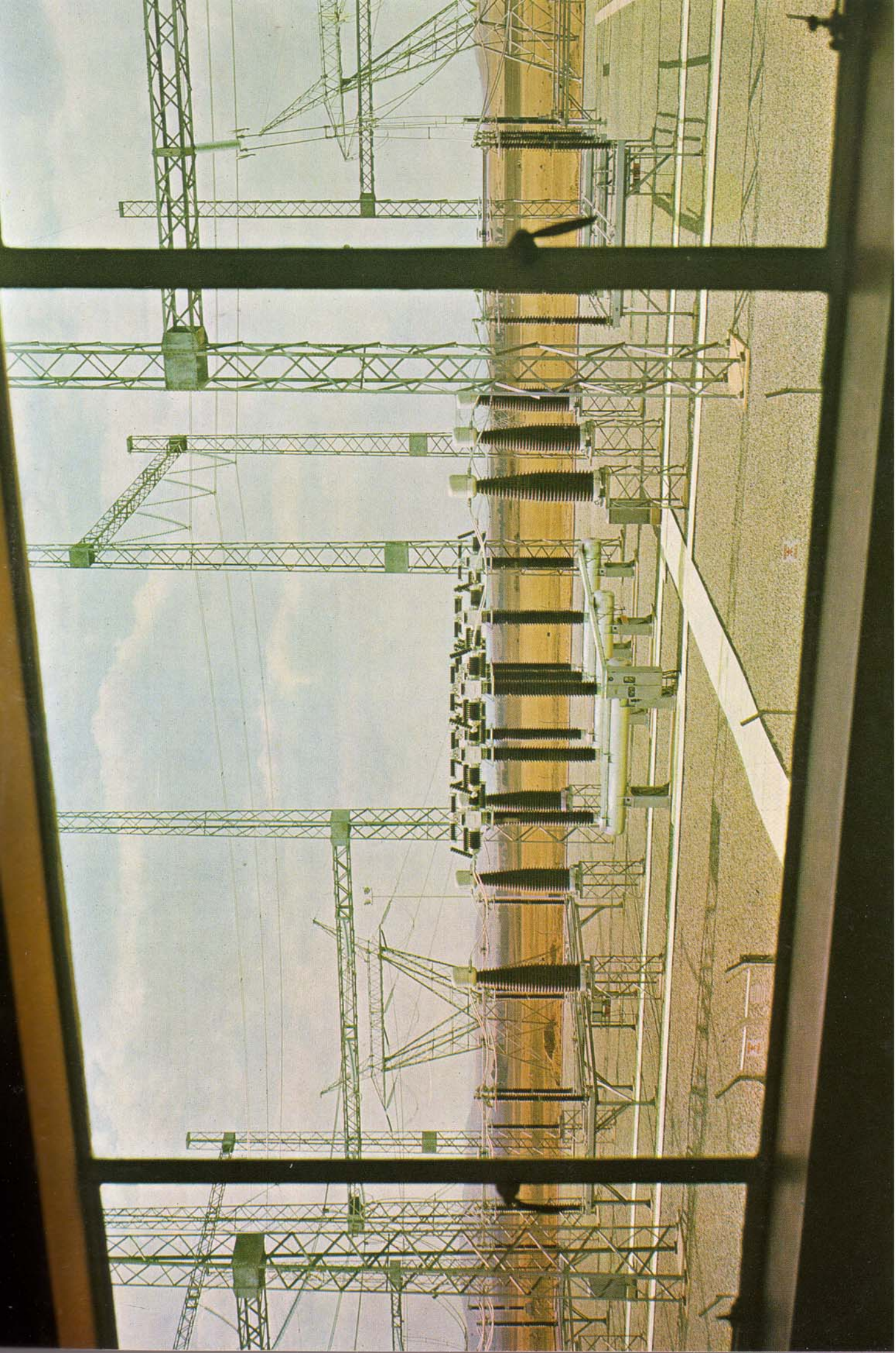
A view of the switchyard at the Atlas distribution station with the incoming 400 kv lines from Camden.
