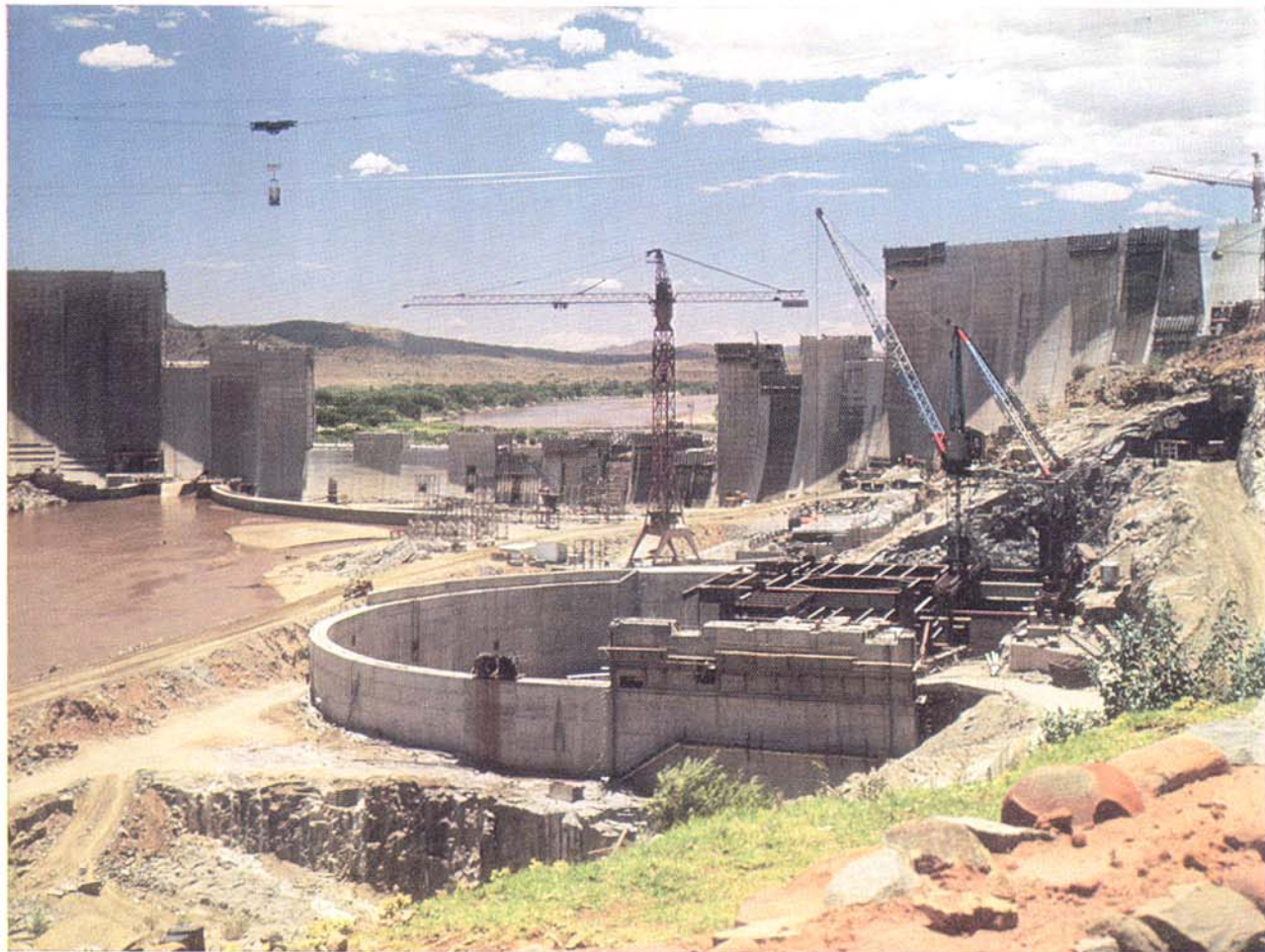
Work is proceeding apace on Escom's hydro station (in the coffer dam in the foreground) at the Hendrik Verwoerd dam. Installation of equipment at this station commenced earlier this year.
