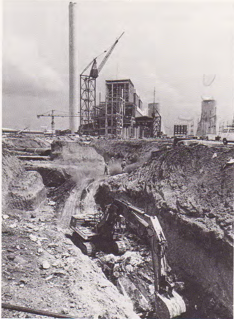
Duyha, a 3 600 MW coal-fired power station under construction near Witbank. Power from here will be fed into Escom's national transmission grid, serving the entire subcontinent.
