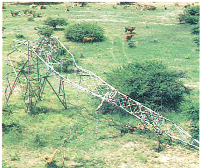
A pylon, pulled down by floods in the Eastern Transvaal. About 30 km of overhead lines were damaged and 53 transformers washed away. In the Cape, the situation was aggravated by snow in isolated mountain areas.
