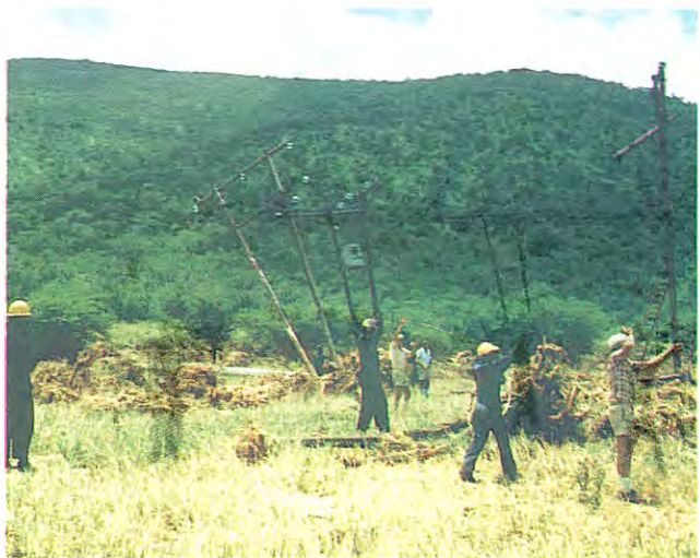
Repair teams busy pulling up lines in the Pongola area. Power was restored to all affected areas in about three weeks, and entailed building nearly 50 km of lines on new and old routes and clearing more than 10 km of dense bush.
